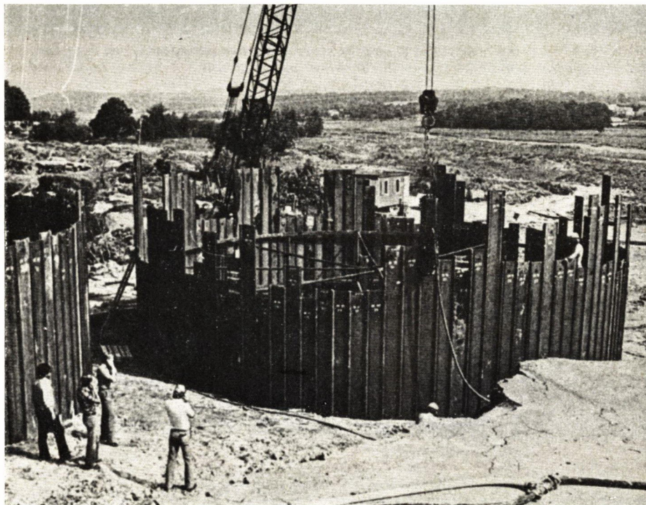
Fig. 27. The circular sheet pile walls were primarily constructed to prevent local stability problems in the clay during placement of the road embankment
