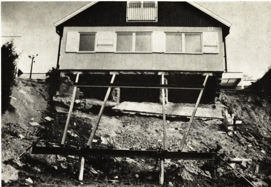
Fig. 7. Temporary struts supporting a building which is hanging over the edge of the slide
